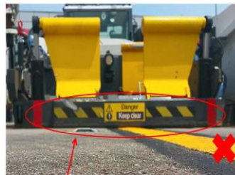
Cradle not fully lifted
